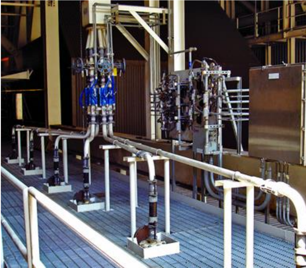
Figure 21. A DSI injection system 46
